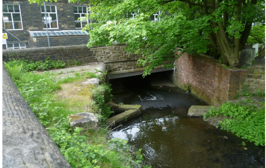
Illustration 1: Structure at risk of blockage
